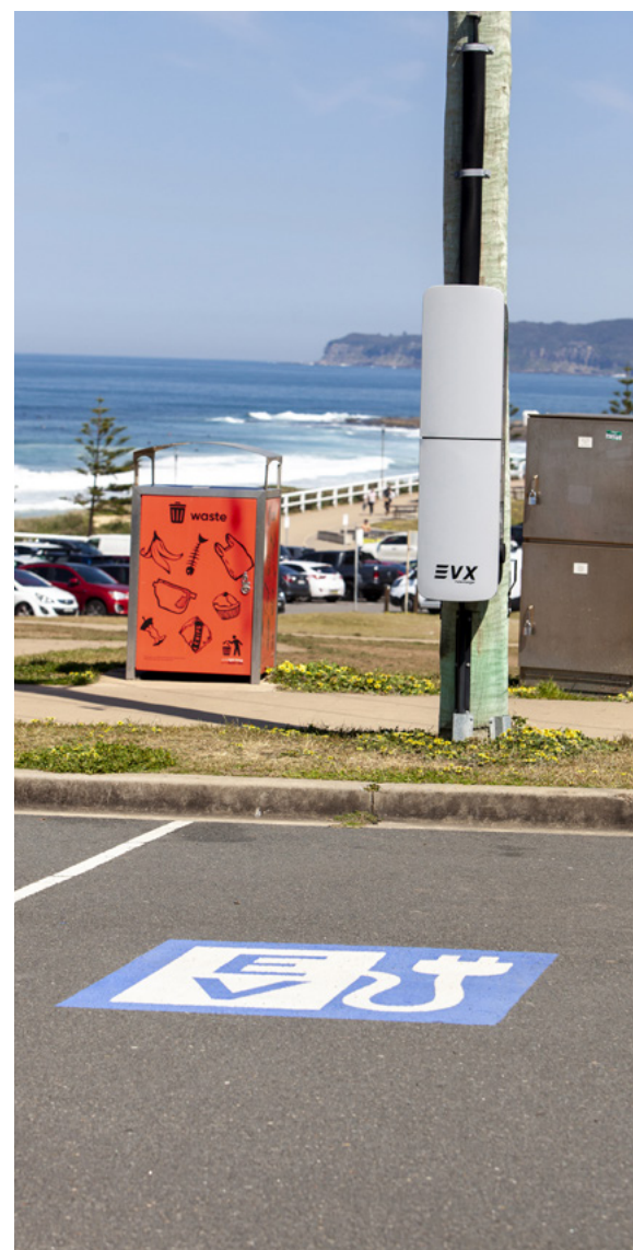
Pole-mounted EV charger at Dixon Park Beach
