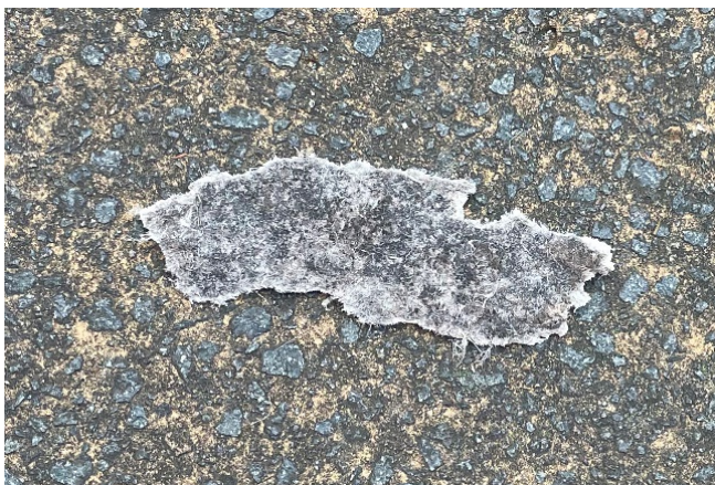
Asbestos debris. Photo: Hazmat Services
