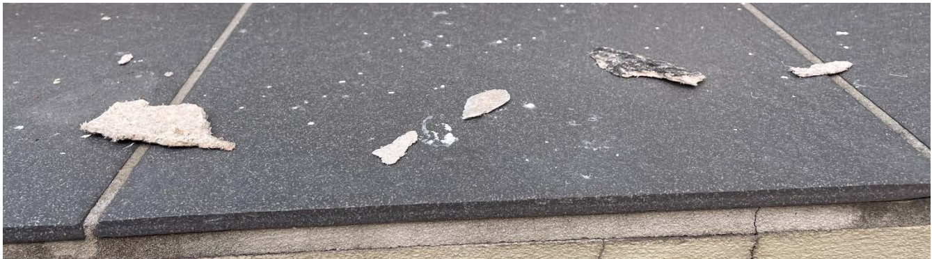
Asbestos debris. Photo: Hazmat Services
