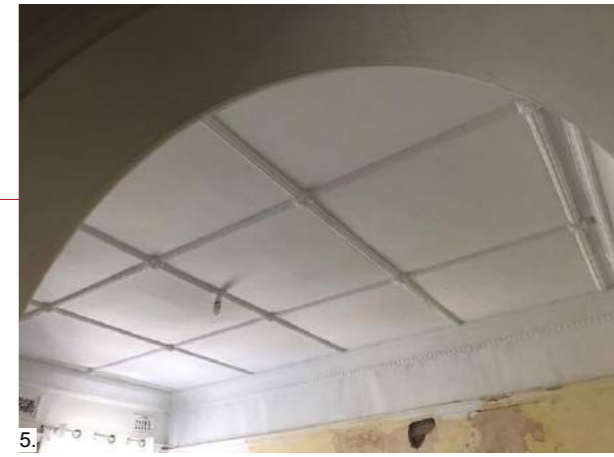
6. REPLACED CEILING WITHIN AFFECTED ROOM. PROVIDING EVIDENCE THAT THIS ROOM HAD BEEN DAMAGED AND REPAIRED IN THE PAST
